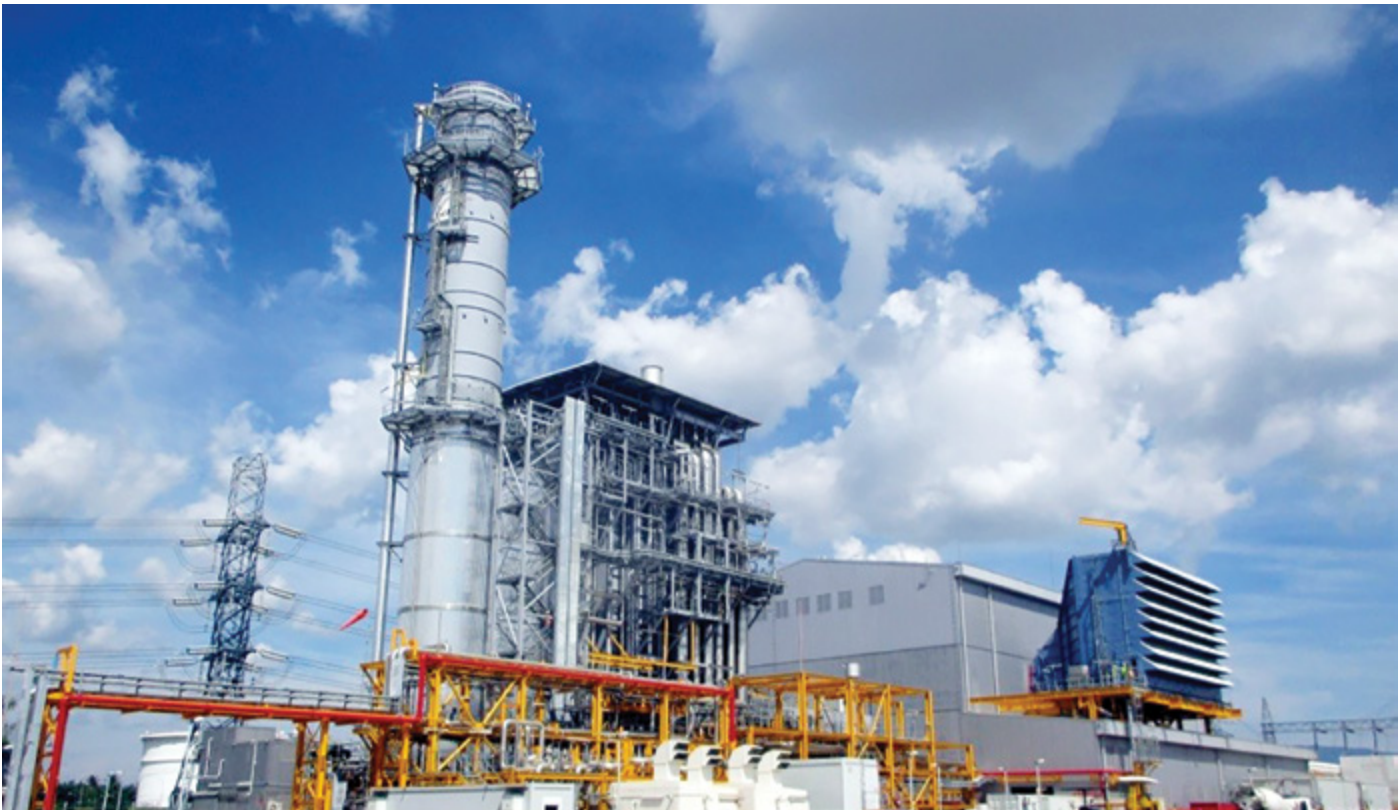
Figure 15. First NatGas Power Corporation (FNPC) operates the 414 MW San Gabriel Power Plant which started commercial operations on November 2016 and is located in the First Gen Clean Energy Complex in Batangas City.
