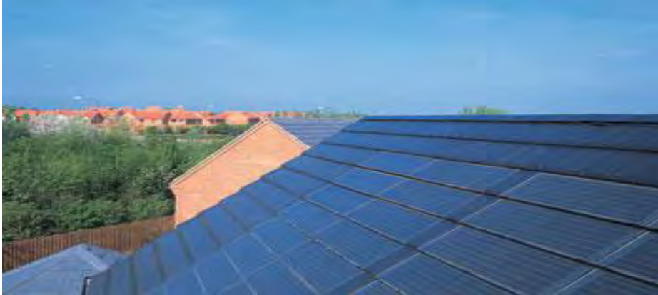
Integrated solar tiles installed by Solar Century on a current development in Milton Keynes by English partnership and Bloor homes
