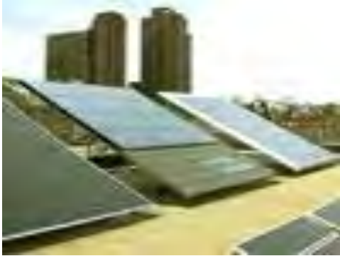
Roof mounted solar panels (Solar century)
